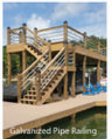
Galvanized Pipe Railing
